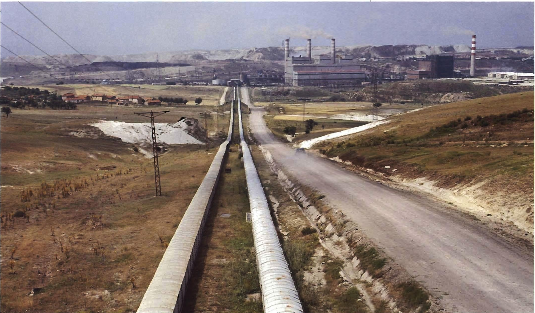
▲ Ash Conveying Belt / ST - 1800 / 1000 mm
