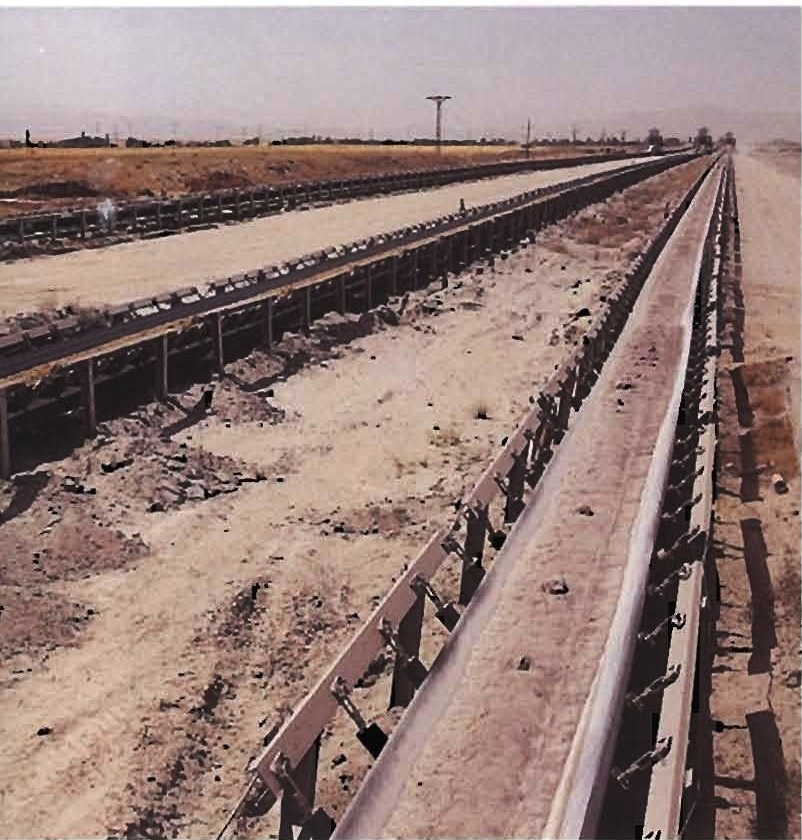
▲ Ash Conveying Belt / ST - 2000 / 1600 mm
